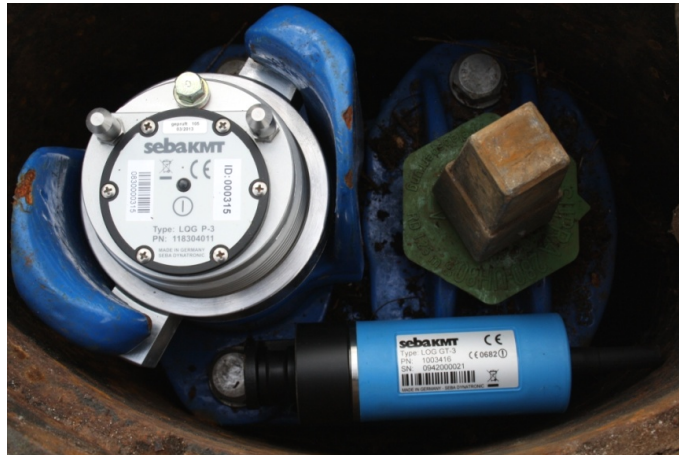
Log P-3 pressure logger and GSM transmitter in a German underground hydrant.
