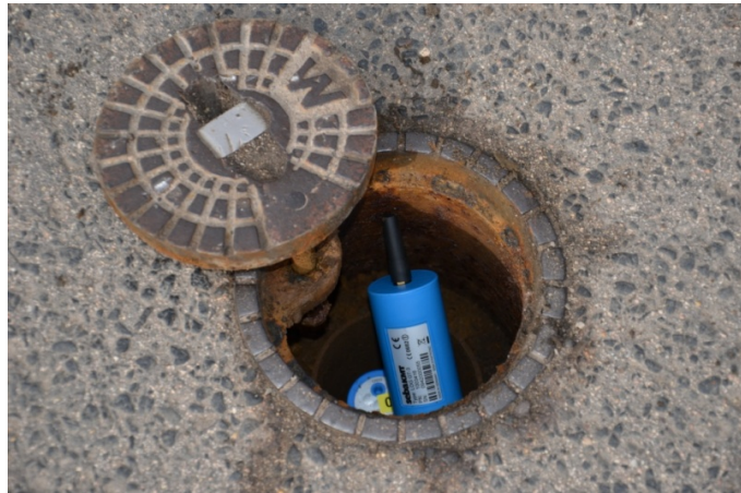
Log N-3 noise logger and GSM transmitter in a German gate shaft.
