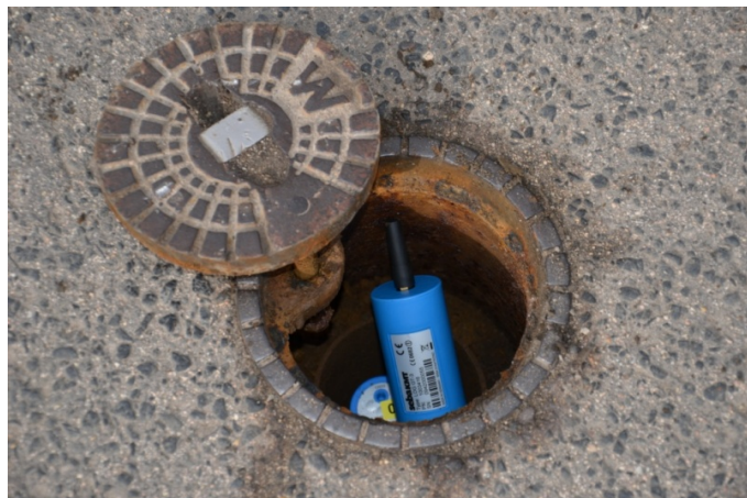
Log N-3 noise logger with GSM transmitter in a German gate shaft.
